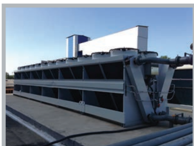
free cooling chillers
