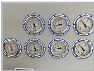
refrigerant and oil gauges
