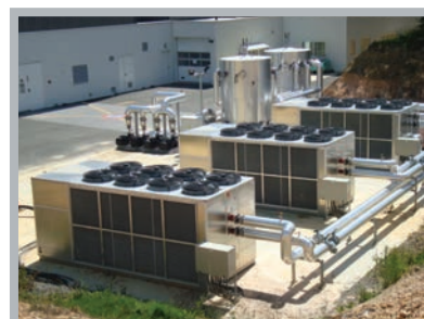
high capacity process chillers
